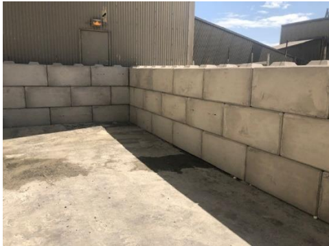
Materials / Aggregate Bunker constructed from interlocking concrete blocks with grout tubes and reinforcing steel
